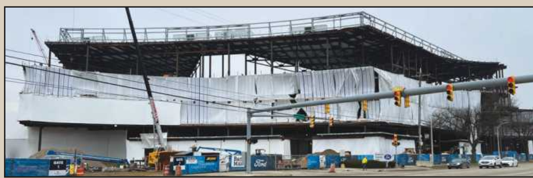
FORD MOTOR CO.'S new Central Campus Building is being erected along Oakwood Boulevard in Dearborn, by Barton Malow and a host of subcontractors. The building, which will house about 6,000 employees, will front a revamped Research and Engineering campus for the automaker..
