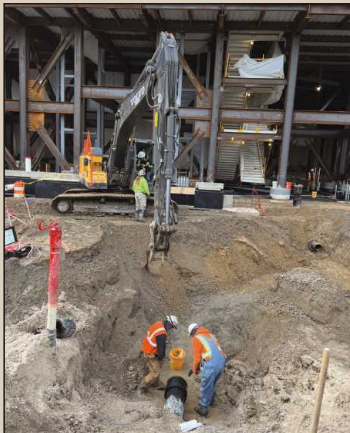
SETTING 10-INCH HDPE fire suppression lines in front of the Ford Central Campus Building are Connor Gestro and Jim Neal of Sprinkler Fitters Local 704. They're employed by Progressive Mechanical. With them are Laborer Travis Childress of Local 1076 and Kevin White of Operating Engineers Local 324, working the excavator.
