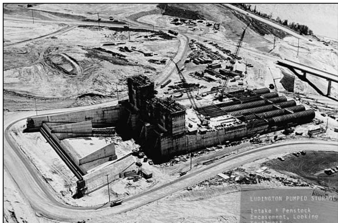
DURING CONSTRUCTION in the early 1970s, shown uncovered are the intake and penstock encasement at the Ludington Pumped Storage Plant.
